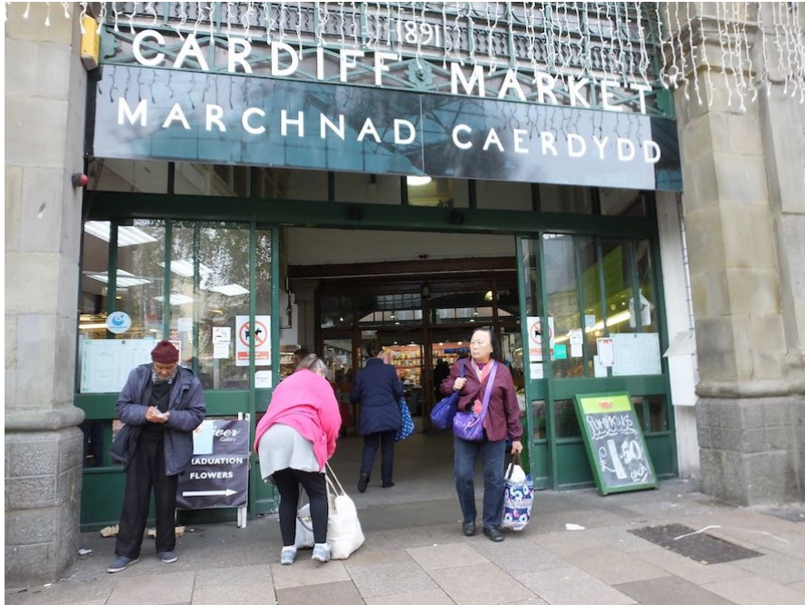
Entrance doors. Recently applied Welsh signage is a distraction from the cast iron tracery. Doors to be replaced and ironwork above refurbished.
