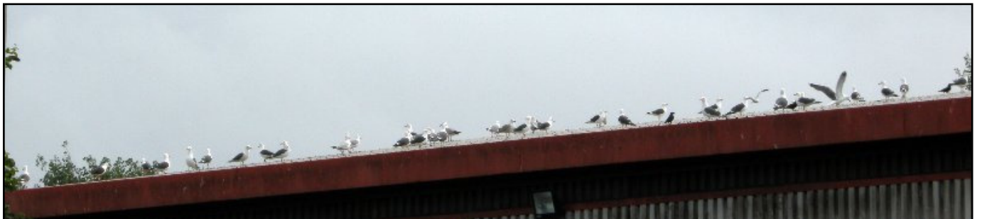
Part of the Biffa transfer station roof at the end of Bessemer Close.
